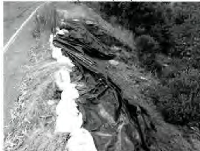
Grizzly Peak Blvd is being undermined by erosion
